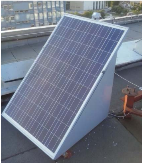
Fig.1. A view of the fixed mount photovoltaic system installed on the roof of the Poznań University of Technology building
