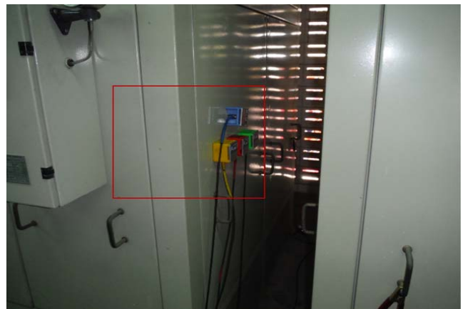
Fig. 12. The position of partial discharging on transformers.
