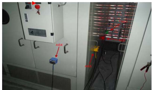
Fig. 8. The installation position of the horizontal axis signal sensor
