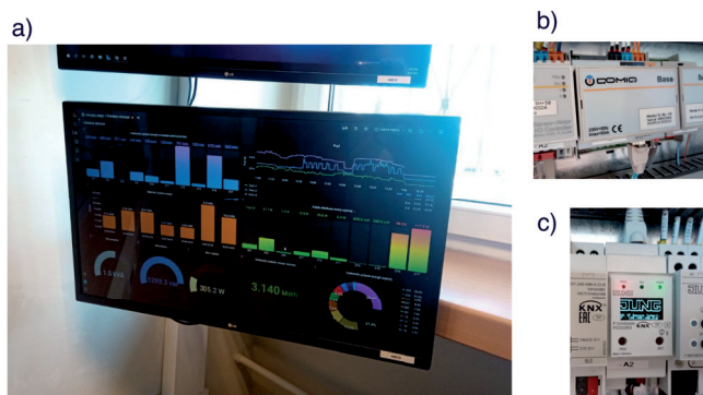
Fig. 6: Real application of InfluxDB working with the Grafana visualization tool (a), retrieving data from the BACS network gateways (b, c) via Telegraf.
