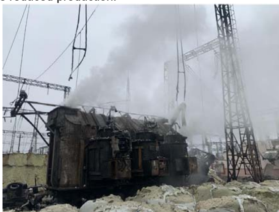
Fig. 1. Damaged power transformer at high-voltage substation.
